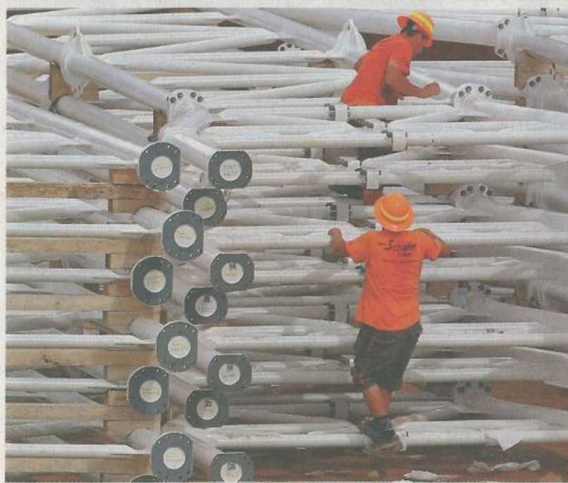
Construction has begun on the Central Waterfront wheel to be operated by Swiss AEX. Photo: David Wong
